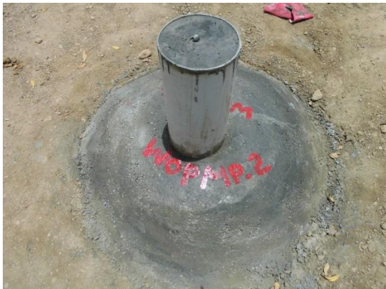
Pipeline Route Marker (Typical)
